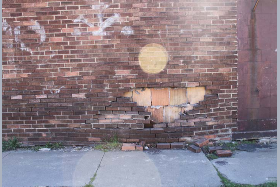
Crumbling buildings in River Rouge may be prevented with proper upkeep and dedicated landlords
