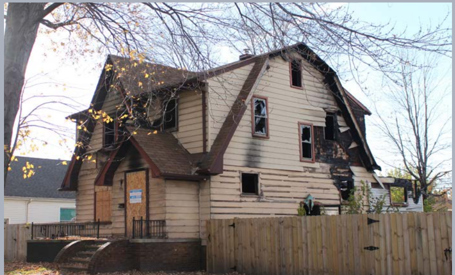
The top housing priority for residents is to demolish blighted structures, particularly those which have been subject to considerable fire damage
